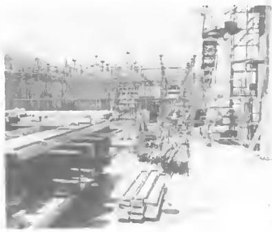
A new building for the museum in the Queensland Cultural Centre. Left : under construction, 1982; below , nearing completion, 1984 — the museum is in the centre of the picture, the windows of the two upper levels looking north across the roof of the art gallery ( centre foreground ).
